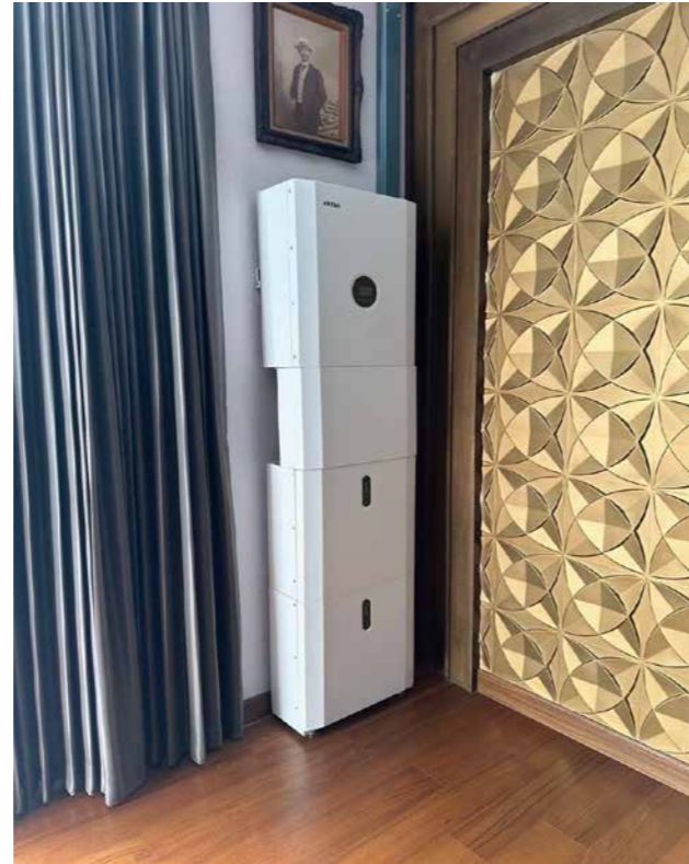
02 Bangkok, Thailand Solar-Powered Home with Battery Storage
