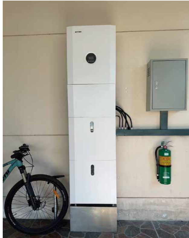
01 Pathum Thani, Thailand Solar-Powered Home with Battery Storage
