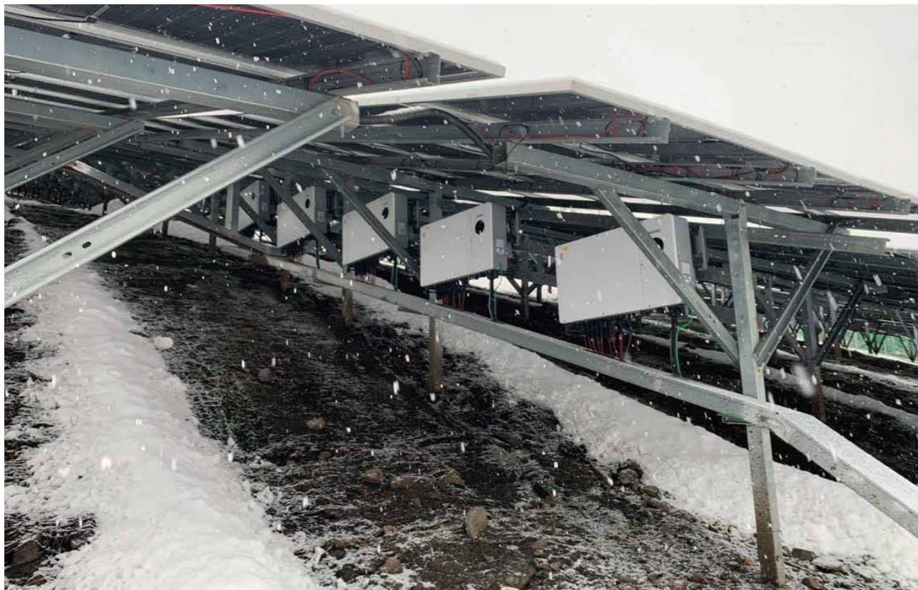
09 C&I Project in Gimhae, South Korea 5MW, KSG-110CL-C1-I25
