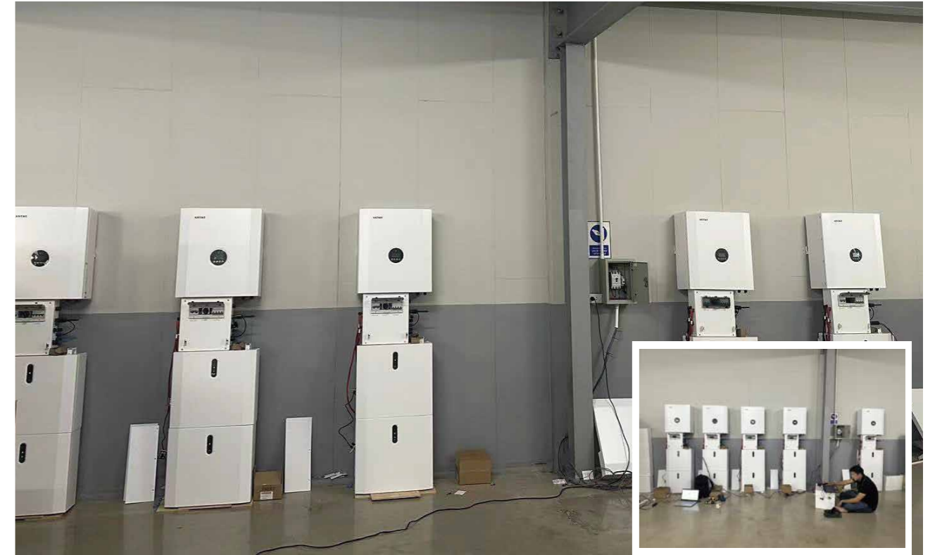
04 Bangkok, Thailand Solar-Powered System with Battery Storage
