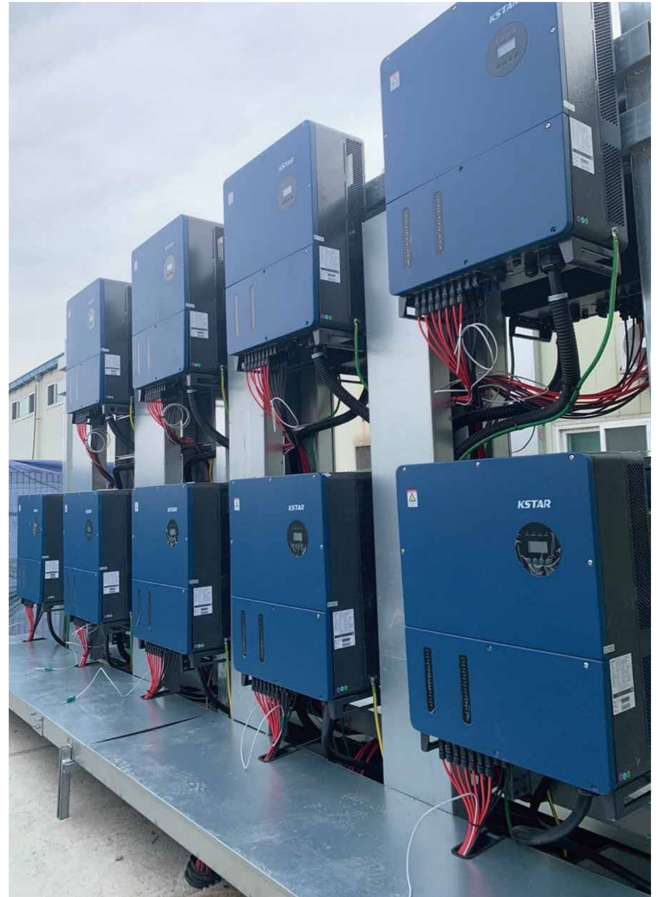
10 C&I Project in Daejeon, South Korea 1MW, KSG-60K-A
